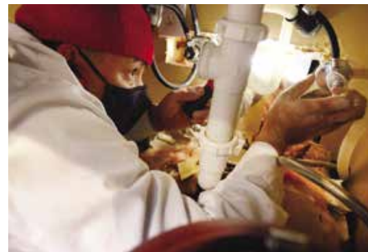
(BOTTOM) Contractor Geovanni 'Geo' Marino of Baker Brothers Plumbing repairs a broken water pipe under Joe Ellery's kitchen sink.
