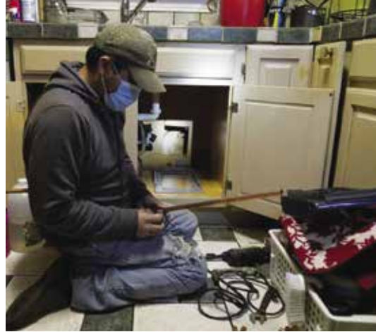
(TOP) Contractor Roberto Valerio works on repairing a broken pipe in the home of Nora Espinoza in Dallas. The pipe broke during freezing temperatures brought on by winter weather.
